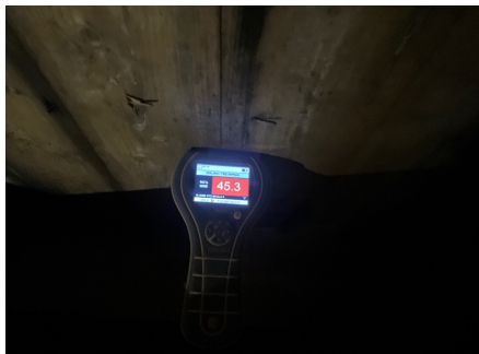
fritt vann i undertaket.
