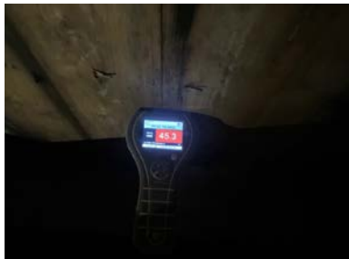
fritt vann i undertaket.
