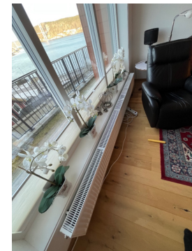
Stor radiator i stue under vindu
