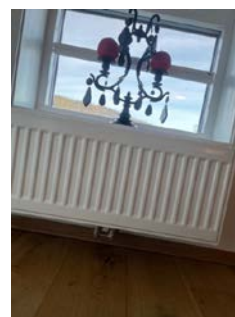
Mindre radiator i stue under vindu
