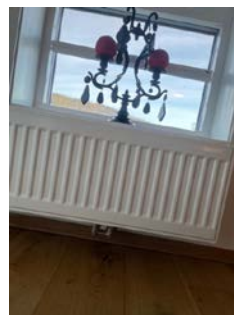
Mindre radiator i stue under vindu
