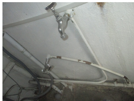
Eldre slitt vvs opplegg
