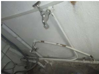
Eldre slitt vvs opplegg
