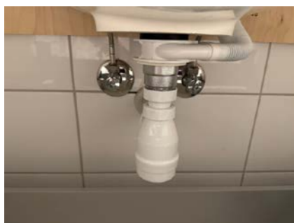
Rørproppleg under servant.
