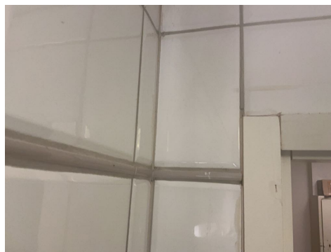
Sprekker i fuger.
