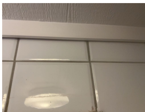
Sprekker i fuger.
