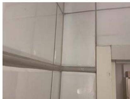
Sprekker i fuger.
