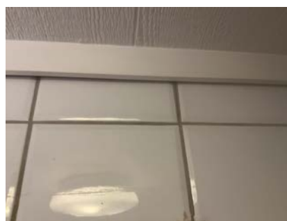
Sprekker i fuger.
