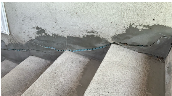
Sprekker i puss over betongtrapp.
