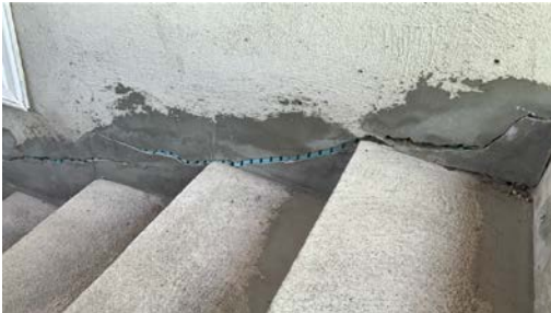
Sprekker i puss over betongtrapp.
