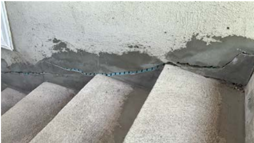
Sprekker i puss over betongtrapp.
