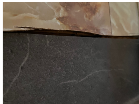
Glippe, hull i vegg.
