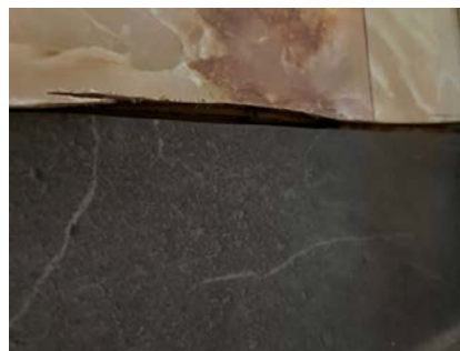
Glippe, hull i vegger.
