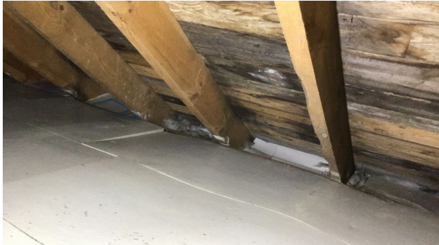
Fukt i undertak
