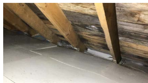
Fukt i undertak
