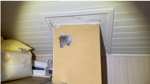
Sprekker/riss i pipe/puss.
