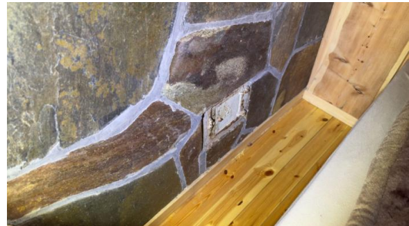
Manglende ildfast plate under feieluke.
