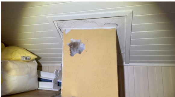
Sprekker/riss i pipe/puss.
