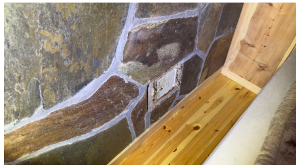
Manglende ildfast plate under feiluke.
