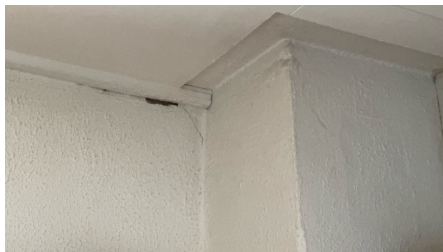
Riss/sprekker i pipe.
