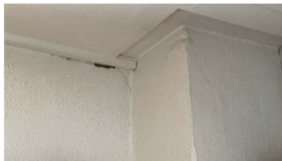
Riss/sprekker i pipe.
