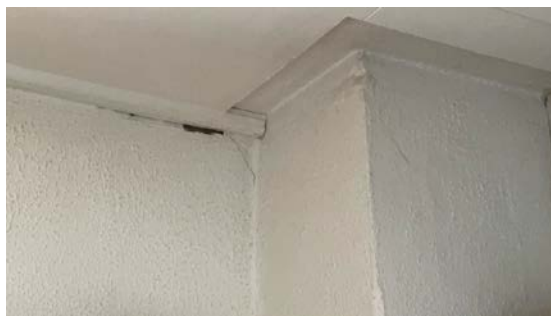
Riss/sprekker i pipe.
