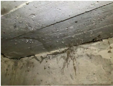
Kondensdråper under himling.
