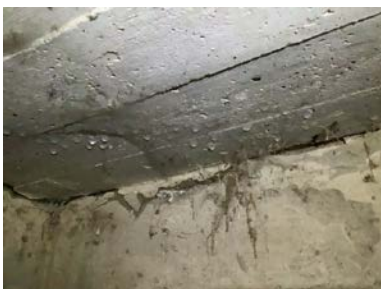
Kondensdråper under himling.
