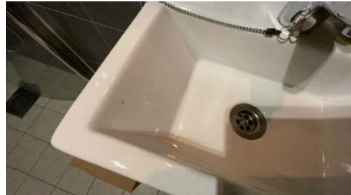
Riss i servant
