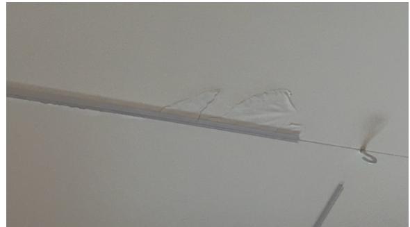
Avskaling i himling.
