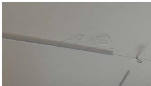
Avskaling i himling.
