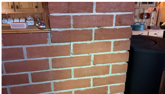
Sprekker i pipe
