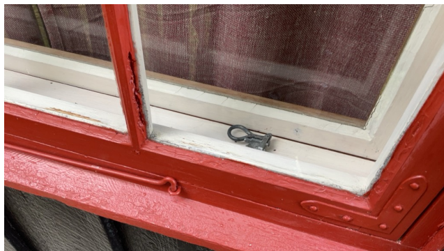
Sprekkdannelse i kitt
