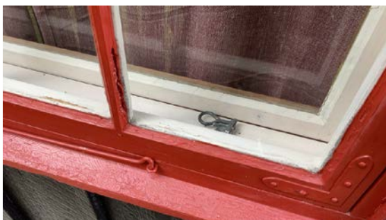
Sprekkdannelse i kitt
