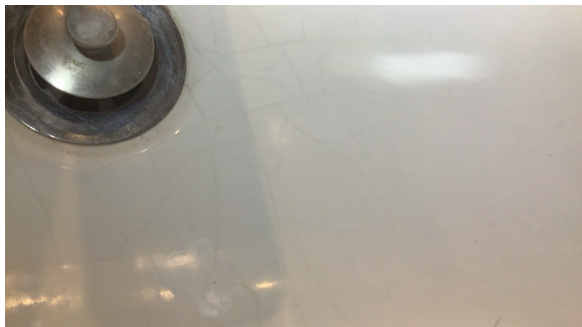
Riss i servant.
