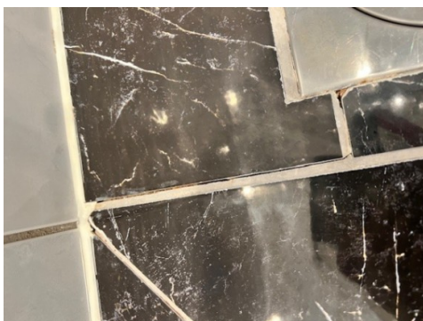
Sprekk/riss i flisefuger.
