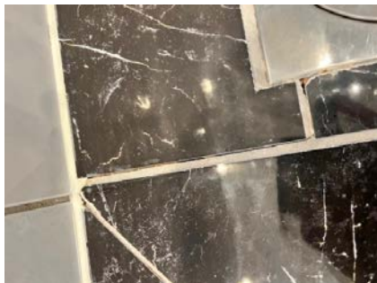
Sprekk/riss i flisefuger.
