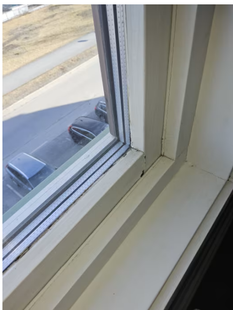
Krakelert maling i vinduskarm.
