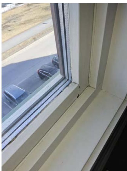
Krakelert maling i vinduskarm.
