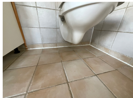
Mangler hull for lekkasjesikring.
