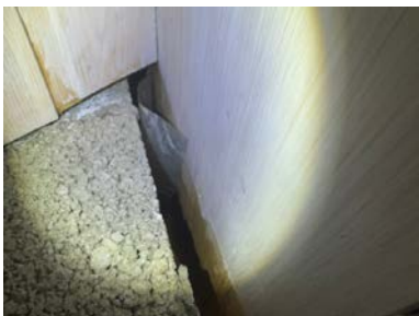
Dampsperran rundt pipen.
