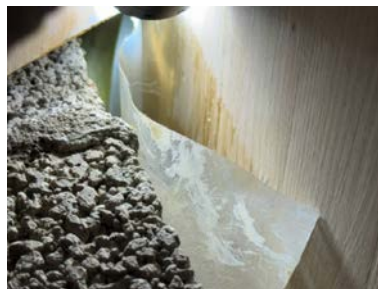
Dampsperran rundt pipen.
