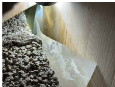
Dampsperran rundt pipen.
