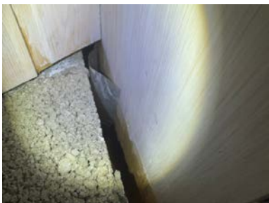
Dampsperran rundt pipen.
