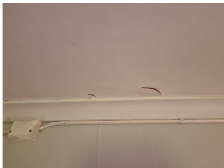
Sprekker i takessplater.
