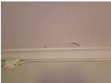
Sprekker i takessplater.
