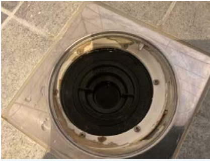
Manglende membran under klemring.
