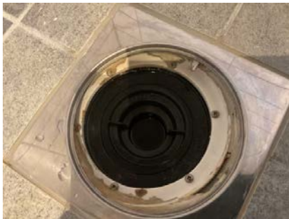
Manglende membran under klemring.
