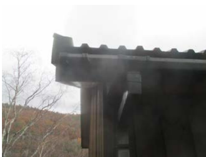
Eldre slitte takrenner.
