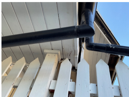
Skjolder i undertak
