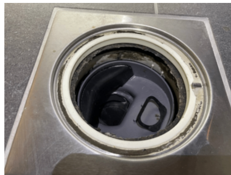
Sluk under benk
