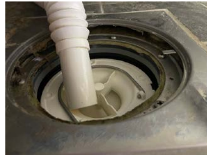
Sluk under kabinett
