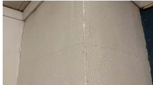
Riss i pipe
