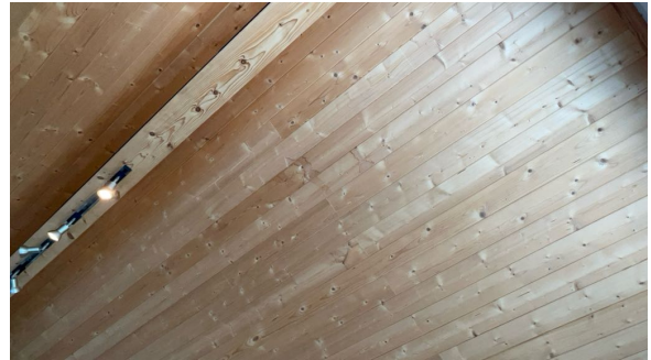
Fuktmerker i himling i stue.
