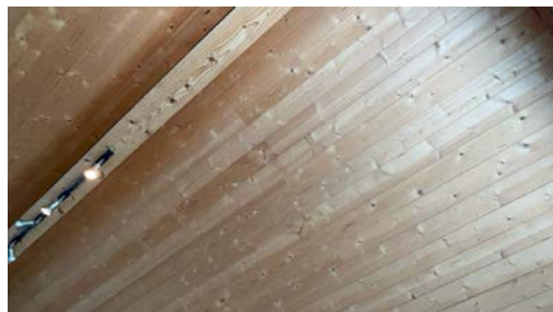
Fuktmerker i himling i stue.
