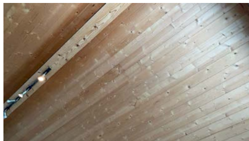
Fuktmerker i himling i stue.
