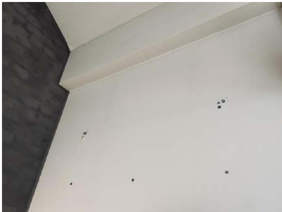
Stedvis plughull i veggoverflater.
